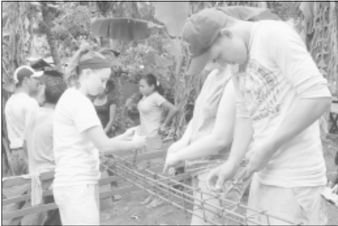
Assembling the rebar which will be used to provide strength and connection for the walls of the parsonage at LaPaz, Carazo.
